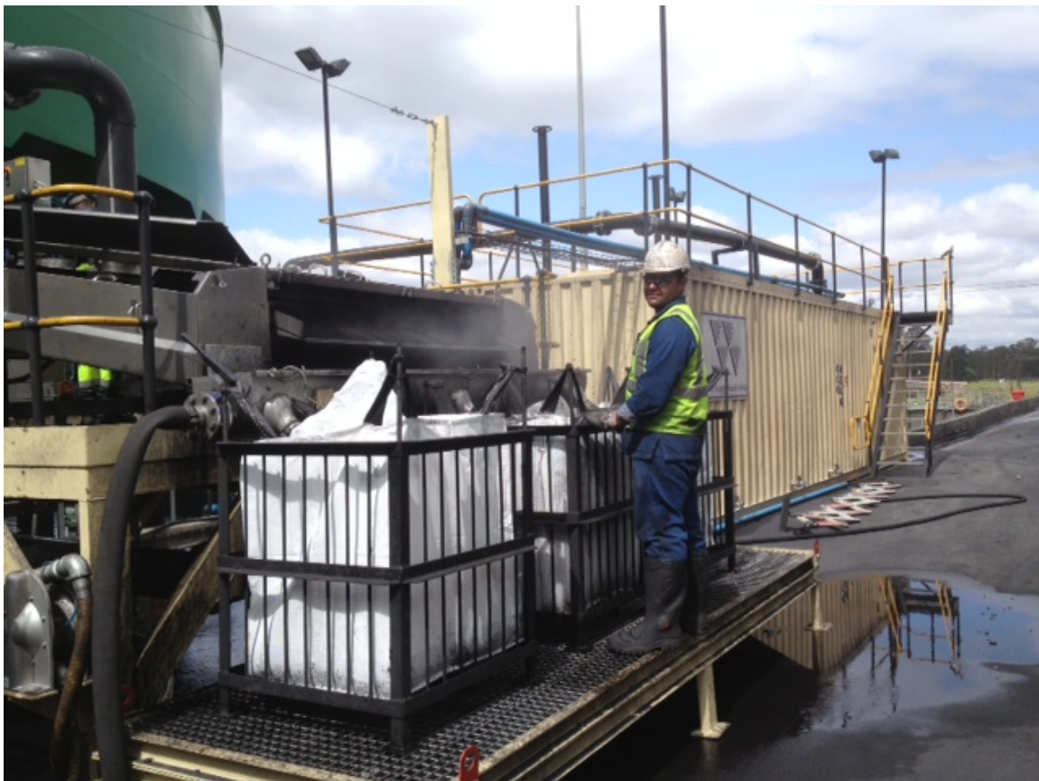
Coal fines screen/filter in operation at a mine site in South Africa, as part of a Detailed Feasibility Study being undertaken by River Energy
