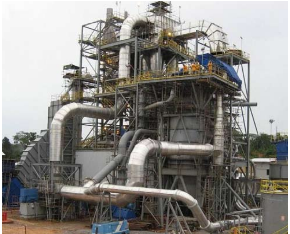
WHITE ENERGY'S CLEAN COAL UPGRADING MODULAR PLANT AT BAYAN'S TABANG MINE IN EAST KALIMANTAN
